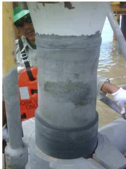
Figure 8. Sample of CUI defect
