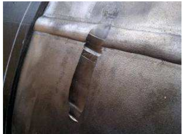
Figure 4. Defect in the 32" pipeline also affecting the seam weld
