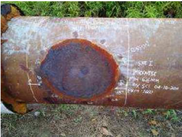
Figure 13. Sample of the CUI defect
